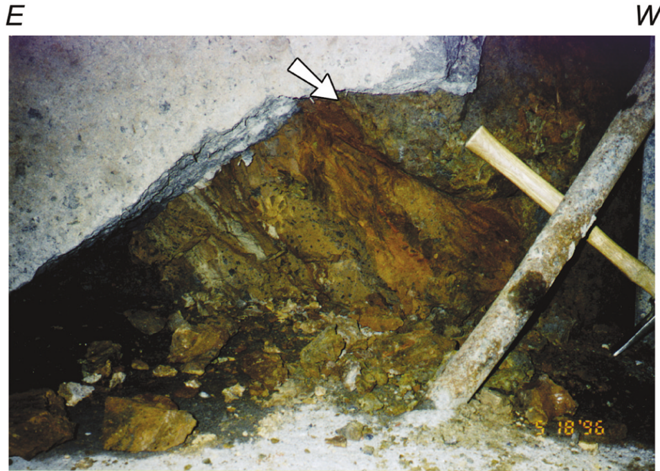
Figure 4. Fault contact inside tunnel. Photograph is of the south wall of the tunnel, approximately 1200 m from the west portal. Arrow indicates a low-angle thrust fault located at the approximate intersection of the tunnel with the mapped trace of the Sylvan fault. Immediately east of photograph, a steeply dipping fault has placed 15-Ma Columbia River Basalt Group above 1-Ma Boring Lava. Gray block in the upper-left corner is construction material.
